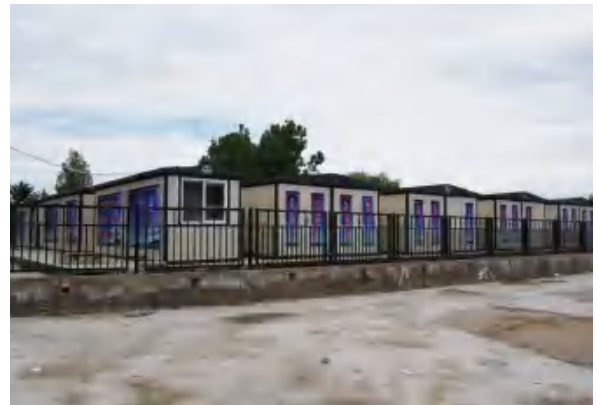
Tongjiafen Rural Centralized Heating Shallow Geothermal Heat Pump Station
