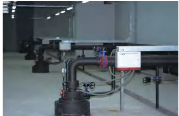
Fig.12 Single Well of Geothermal Energy Collection with Circulation Heat Exchange in the Basement of the National Grand Theatre
