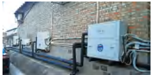
Fig.16 Real Scene of the Outdoor Ground Energy Heat Treasure unit behind the House
