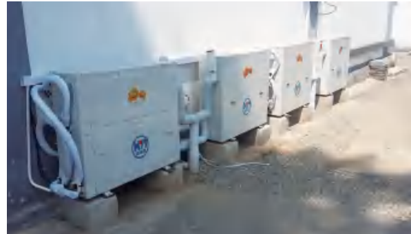
Fig.17 Real Scene of the Outdoor Ground Energy Heat Treasure unit behind the House
