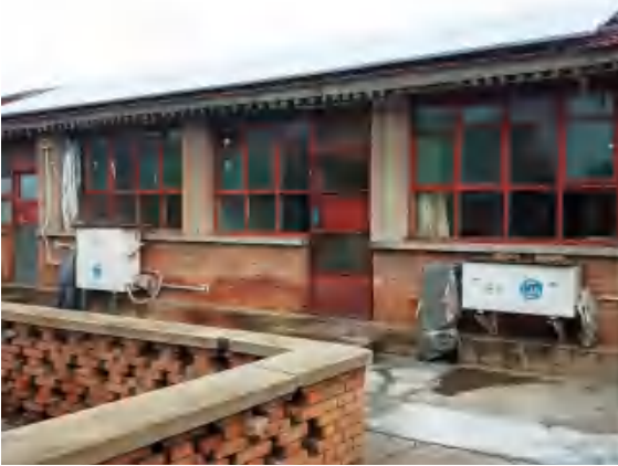
Fig.19 Real Scene of the Outdoor Ground Energy Heat Treasure unit in front of the House
