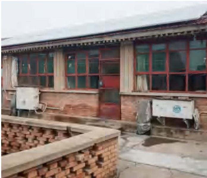
Outdoor unit of geothermal energy heater, rooftop solar power generation
