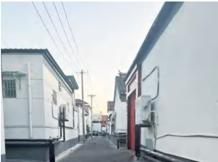
Earth Energy Rebao outdoor unit installed on the exterior wall
