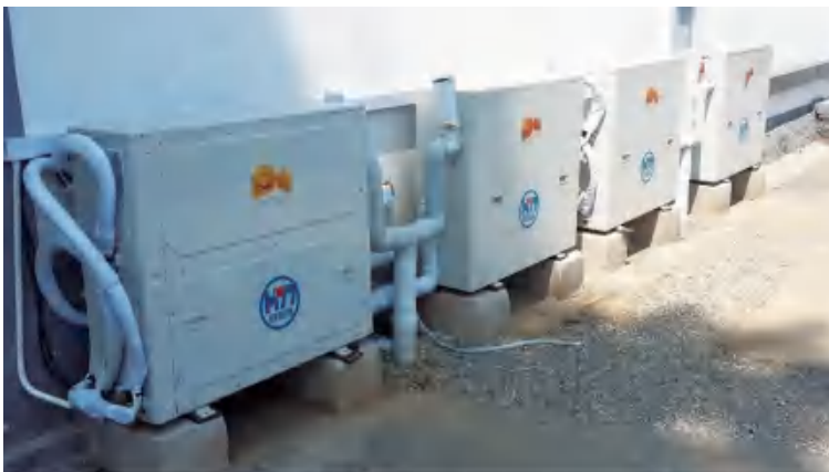
Earth Energy Rebao outdoor unit installed on the exterior wall
