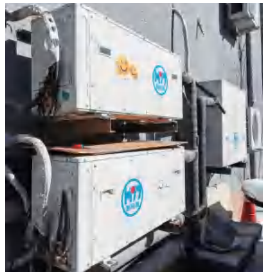
Earth Energy Rebao outdoor unit installed on the exterior wall
