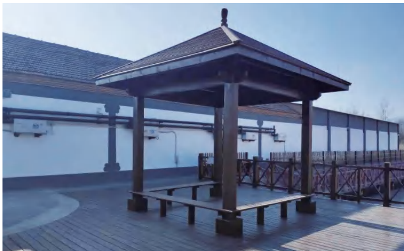
Earth Energy Rebao outdoor unit installed on the exterior wall
