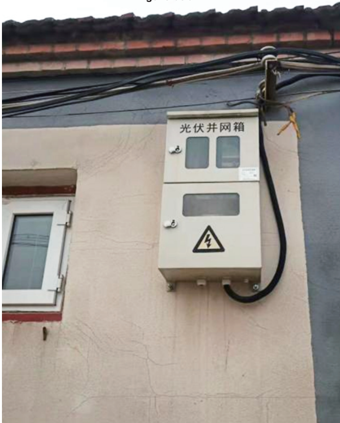
Solar photovoltaic grid connection box
