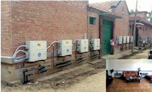
Xizha Village, Shangzhuang Town, Beijing: in the whole village, the efficient electricity was adopted to replace coal, with the heating devices used in each room and metered based on household.
