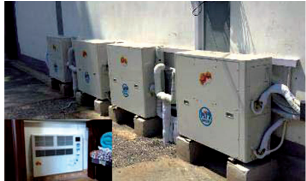
Lijiafen Village, Shangzhuang Town, Beijing: in the whole village, the efficient electricity was adopted to replace coal, with the heating devices used in each room and metered based on household.
